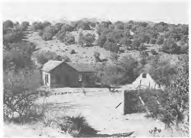
Figure 16. Cabin C (left center) and barn (right). Workers have removed the damaged roof and braced the walls. Photo by Richard W. and Florence B. Lord.
